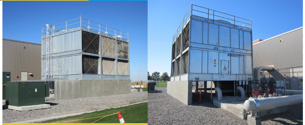
Cooling Towers (photo from Pacific Northwest National Laboratory)
